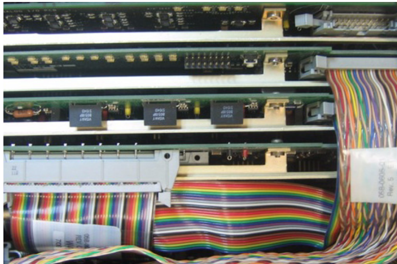
Figure 5-9 Routing of W6 and W7 Ribbon Cables
