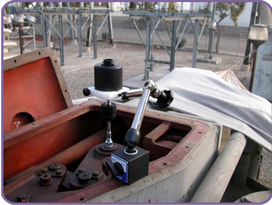
Figure 32. Rotary Transducer on Federal Pacific Breaker
