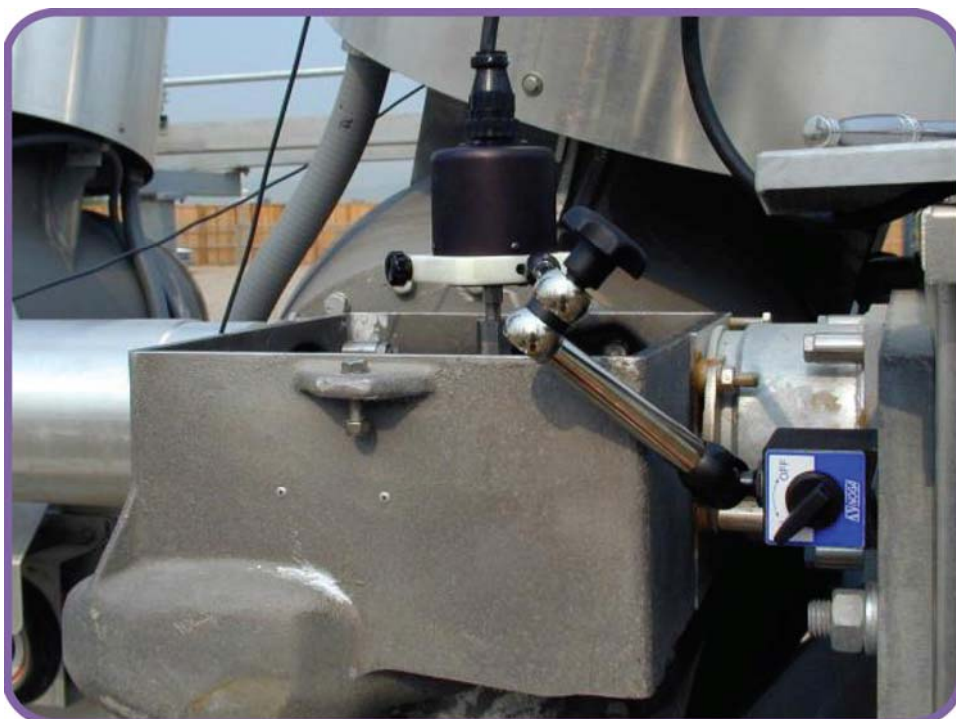
Figure 27. Rotary Transducer on Alstom HE 1014 Circuit Breaker
