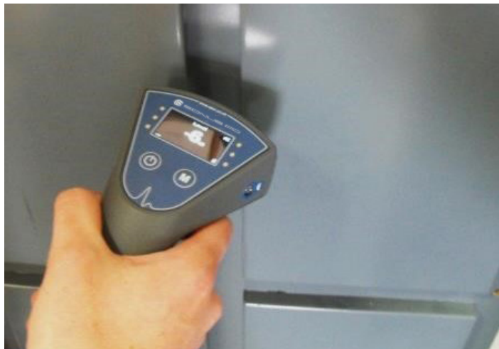
Fig 15: Checking acoustic activity between switchgear panels
