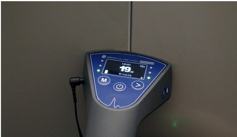
Figure 24: Checking acoustic activity between switchgear panels
